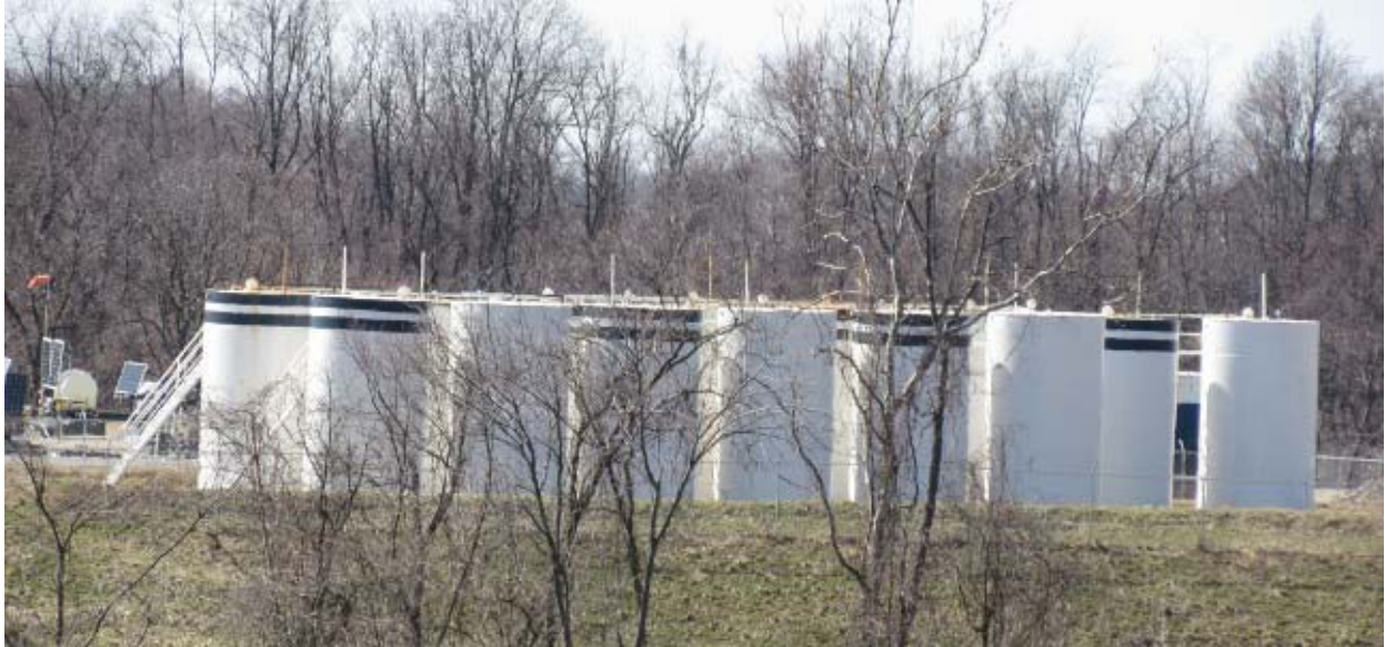
A production field tank battery made up of seven produced water tanks and seven condensate tanks. Tanks are ~400 bbl each.
