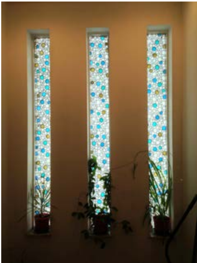
These "hideous plastic-bubbly-window-things" in the GASP office were not energy efficient.
