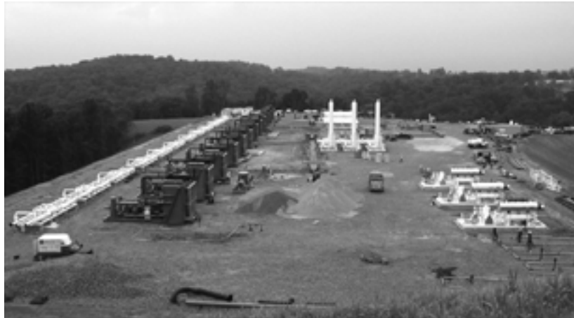
The Pleasants compressor station under construction. Pleasants is one of the two compressor stations that are the subject of the appeal.
