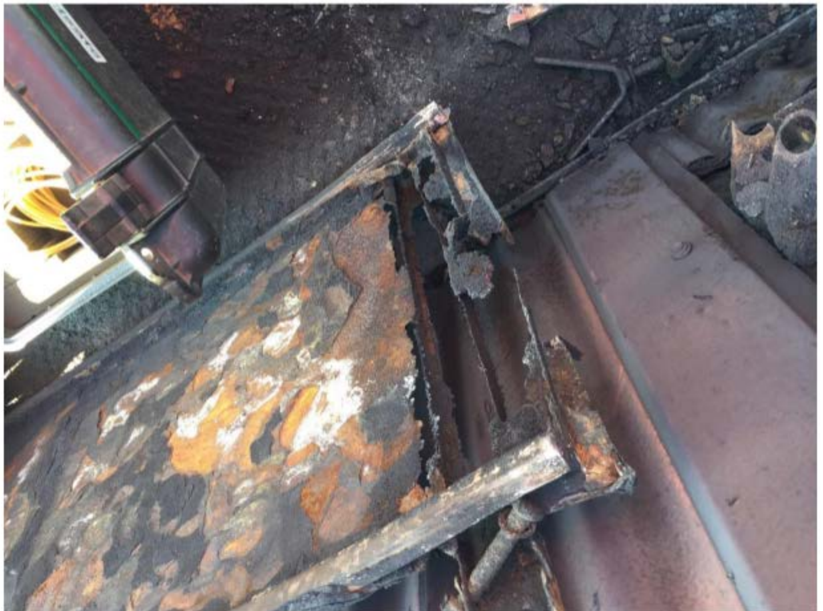
Figure 13 Door Corrosion Door removed from unit
