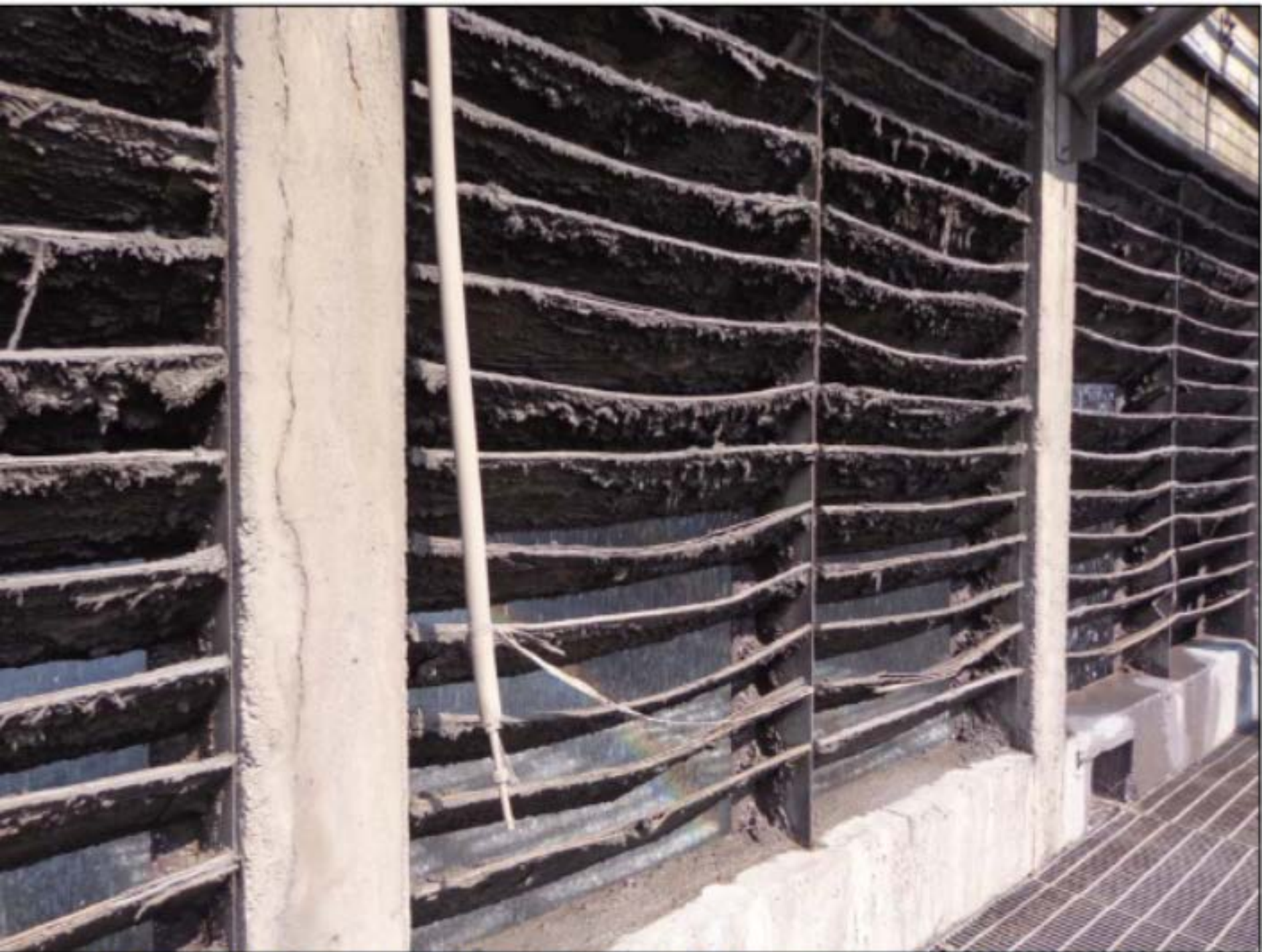
Figure 18: Blast Furnace Recirculation Scrubber Water Cooling Tower louver deterioration.
