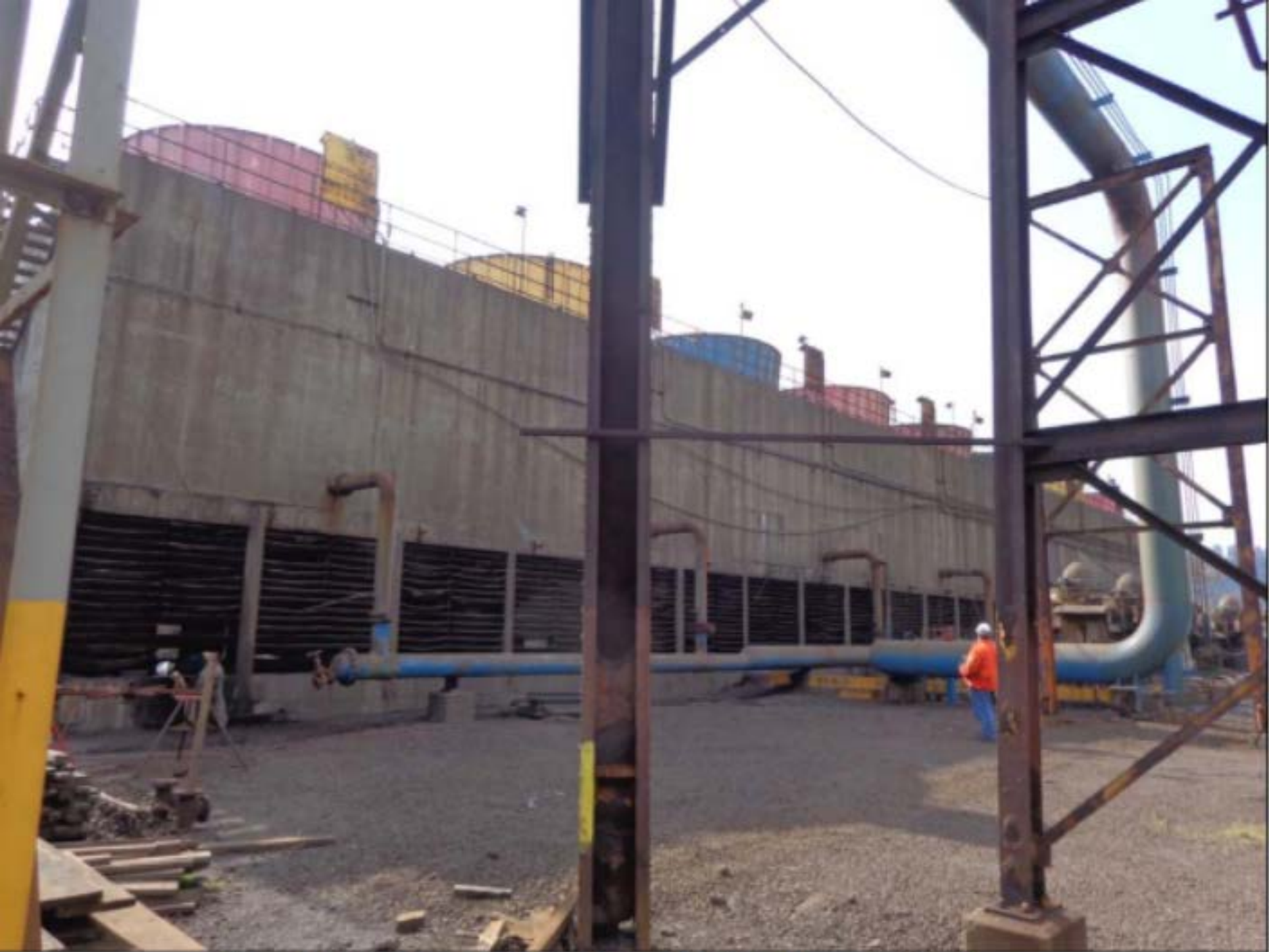
Figure 17: Blast Furnace Recirculation Scrubber Water Cooling Tower.
