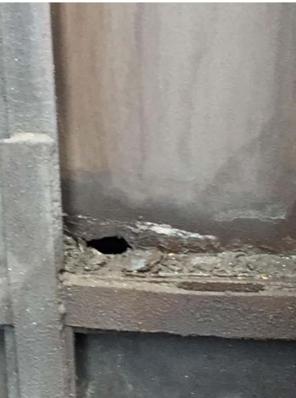
Figure 17 Fan side duct hole
