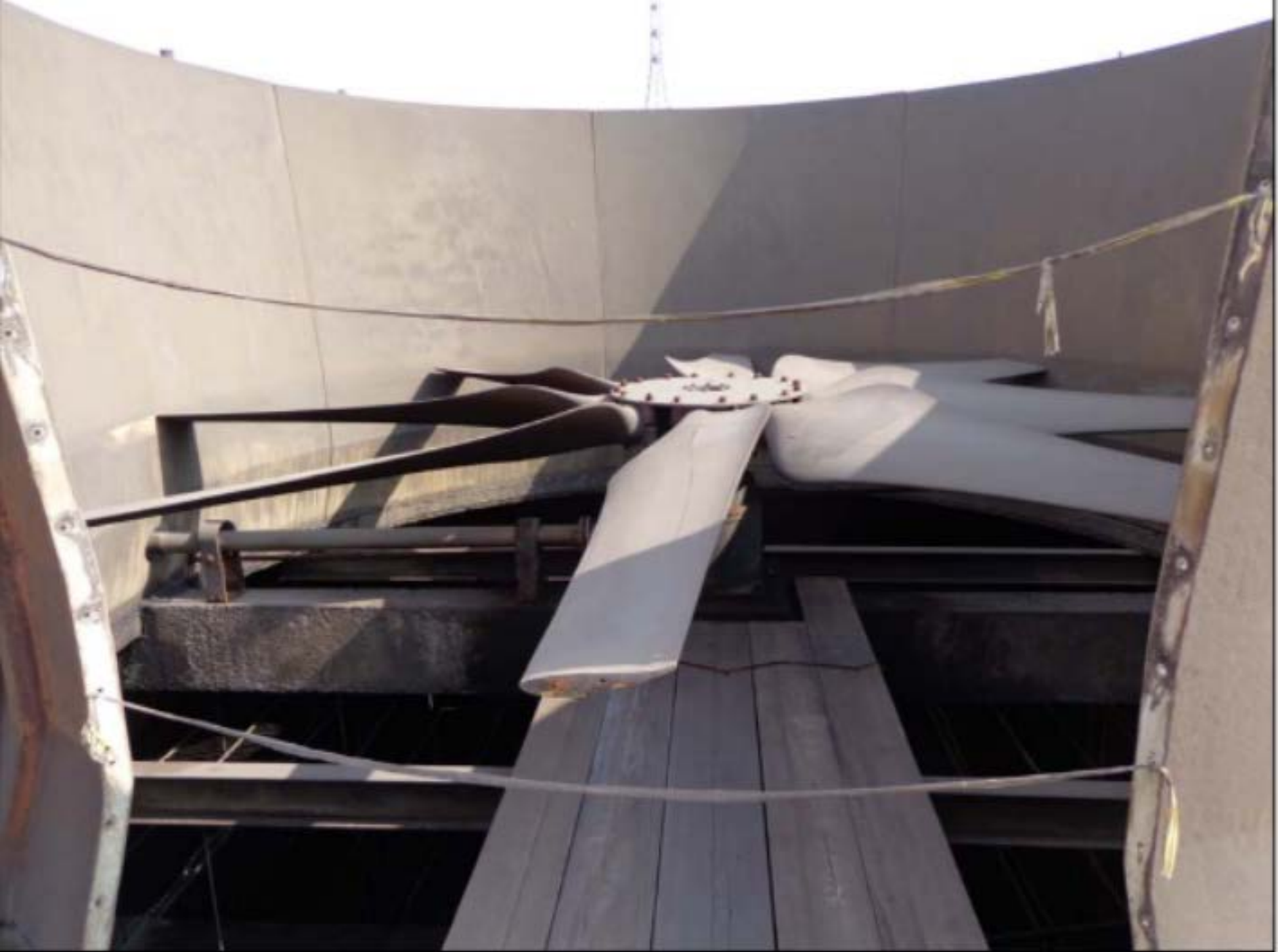
Figure 19: Blast Furnace Recirculation Scrubber Water Cooling Tower fan with leading edge wear and damage. Fan is also missing the center seal disk.
